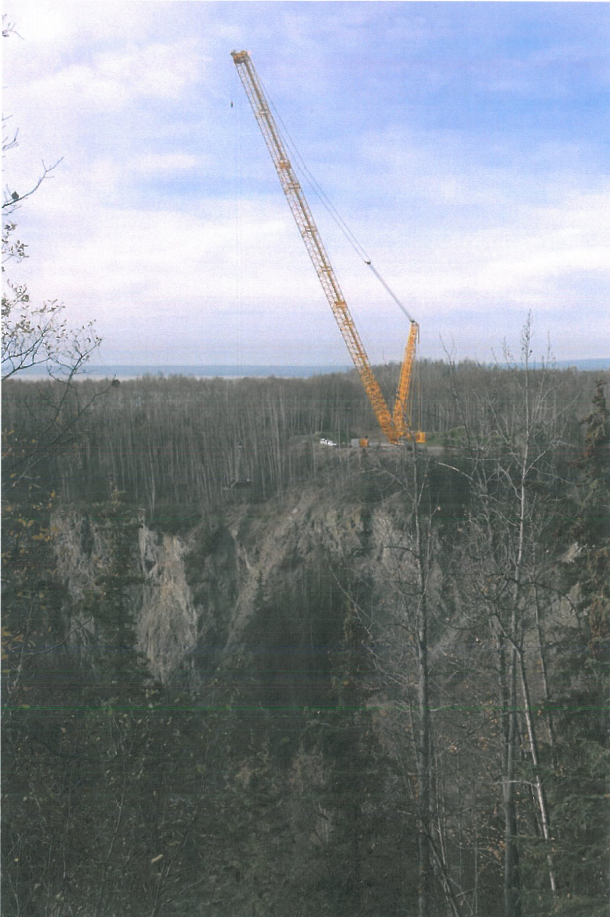
With a 400-foot boom, the crane used in the Eklutna River dam removal project is the largest in Alaska. Photo by Frank E. Baker
