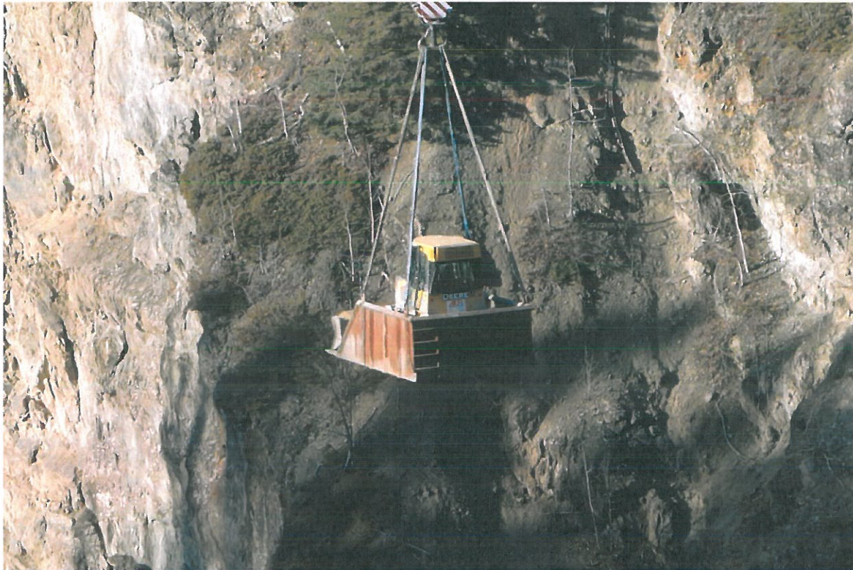
One of the bulldozers used to create a work space for the dam removal next year is hoisted by crane from Eklutna Canyon. Photo by Frank E. Baker
