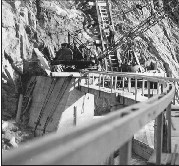
Figure 33. Maintenance work at the diversion dam. Tram in background. April, 1945. Courtesy of Ray Kozlowski.
