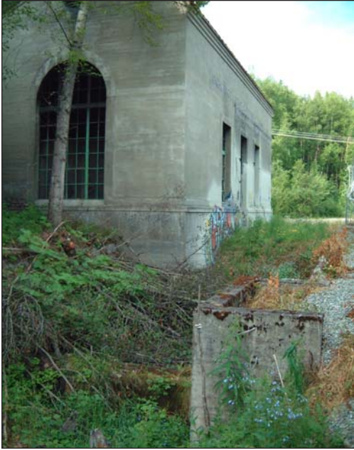
Figure 43. Side and rear view of powerhouse. Tail-race remains in foreground. Photo by R. Sackett, June 2001.
