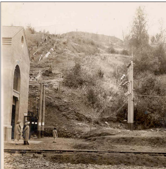
Figure 15. Penstock construction in background behind powerhouse. Note railroad spur in foreground, which was removed after construction was completed.
