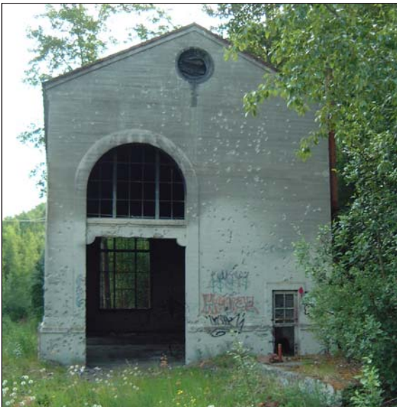
Figure 44. Front view of powerhouse as it appears today. Note that the left lean-to addition (switchroom) is no longer present. Date removed unknown. Photo by R. Sackett, June 2001.
