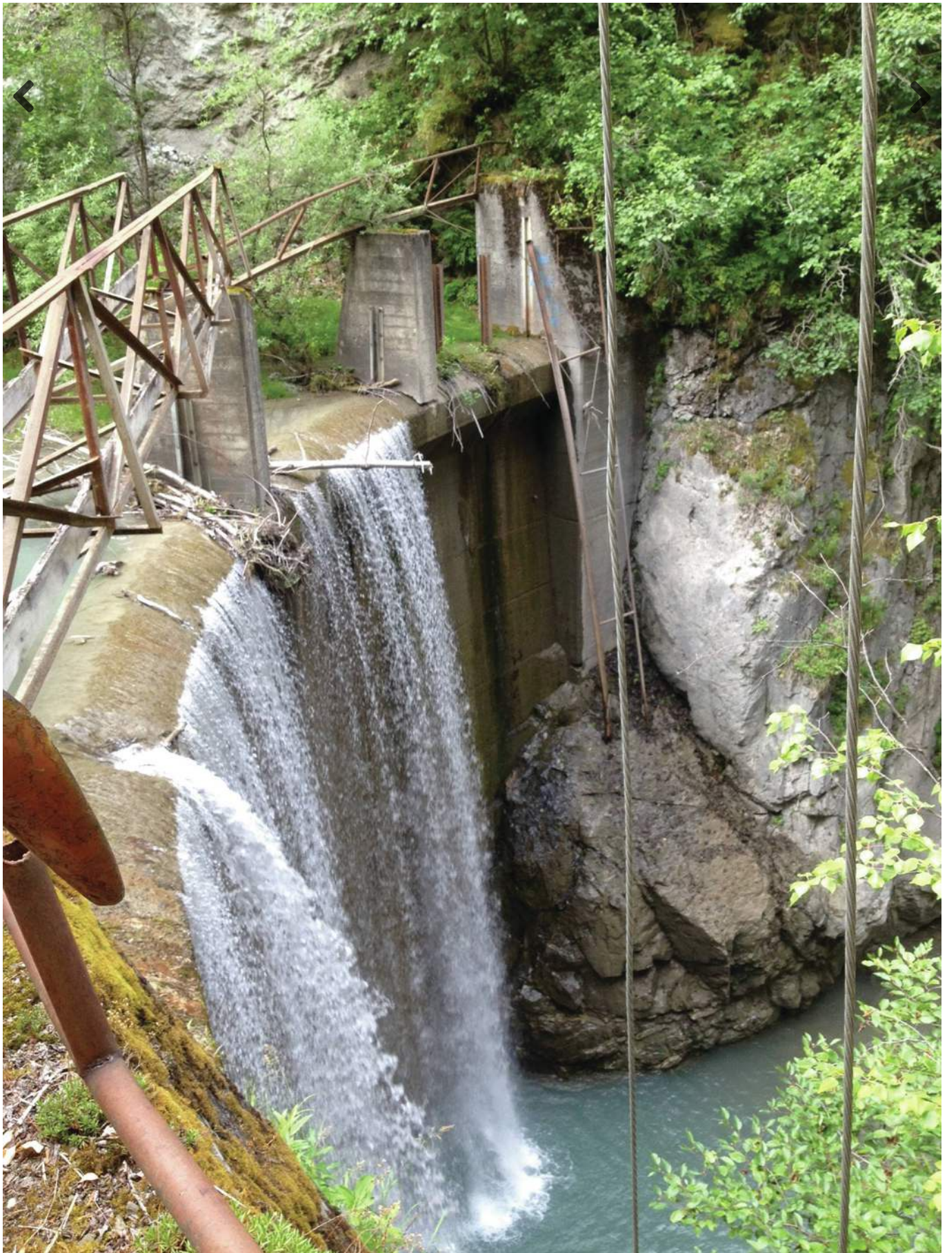
Restoring salmon habitat on the Eklutna River is the goal of demolishing a dam that was built in the 1920s to supply power to Anchorage. (Photo/Courtesy/Eklutna Inc.)
